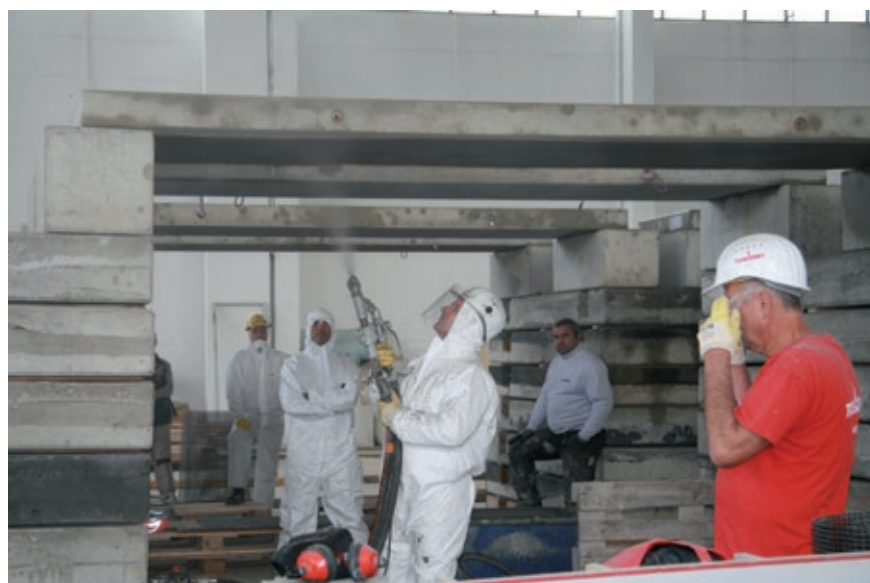
Fig. 3.6: Spraying of next fine concrete layer for preparation of applying next layer of textile reinforcement
